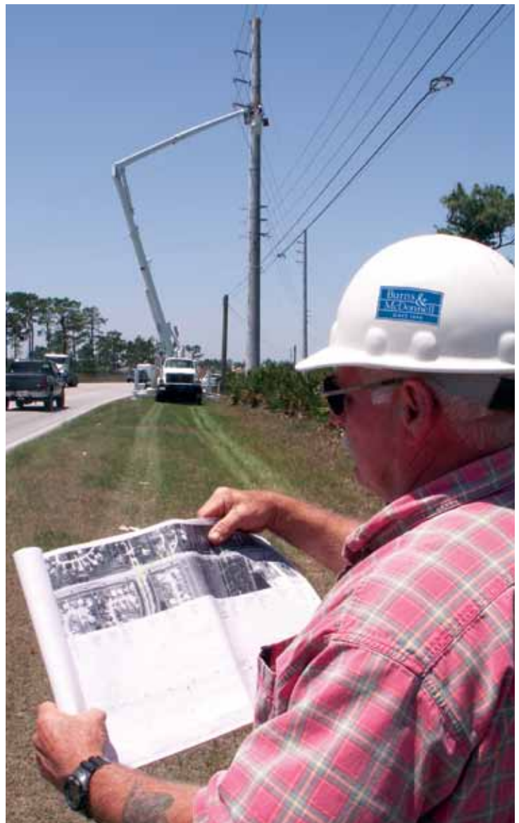
Transmission line impedance is one component to consider when determining fault current magnitude.
